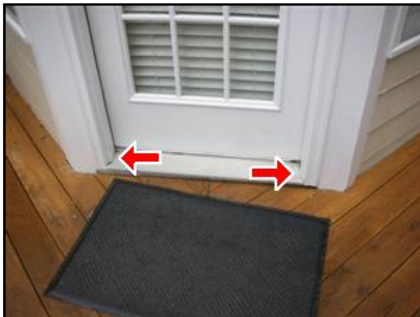
Item 9 - Picture 2 Damaged door jambs
