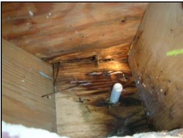
Item 9 - Picture 1 Example of floor system damage
