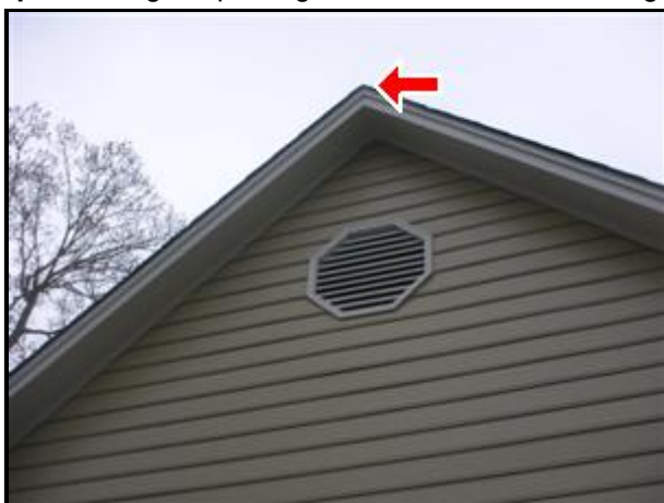
1.0 Picture 1 Torn ridge shingle at front of garage
