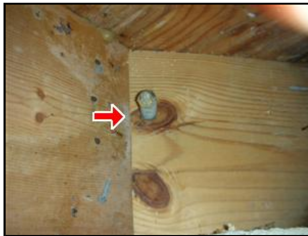
2.3 Picture 1 Example of missing bolt
