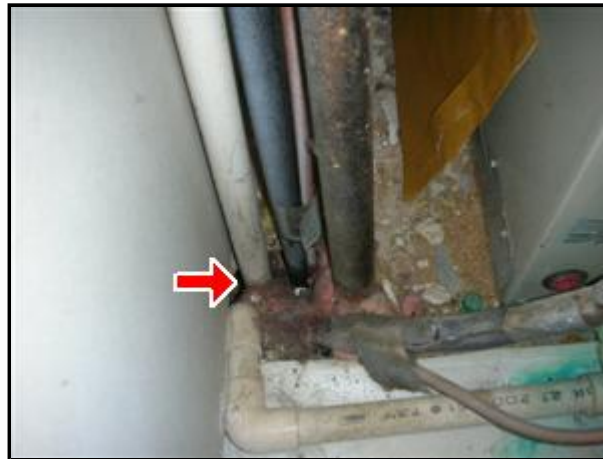
3.2 Picture 1 Gaps to be sealed
