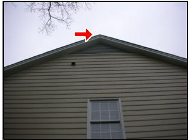
Item 1 - Picture 2 Torn ridge shingle at left gable end
