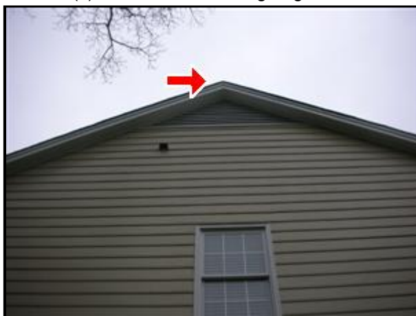
1.0 Picture 2 Torn ridge shingle at left gable end
