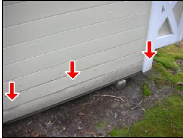
Item 7 - Picture 1 Examples of damaged areas
