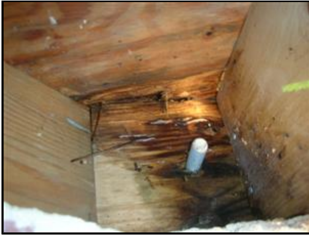
4.3 Picture 1 Example of floor system damage
