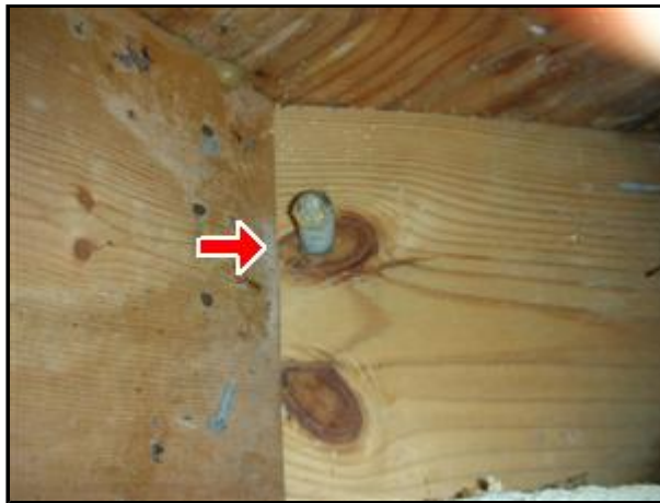
Item 5 - Picture 1 Example of missing bolt
