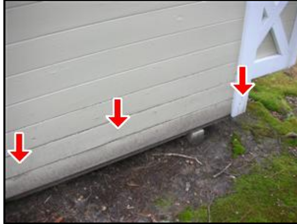
2.6 Picture 1 Examples of damaged areas
